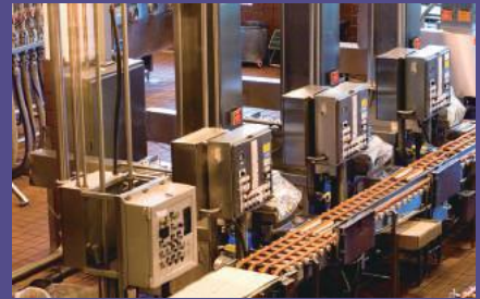
Distributed Monitoring and Control Systems
